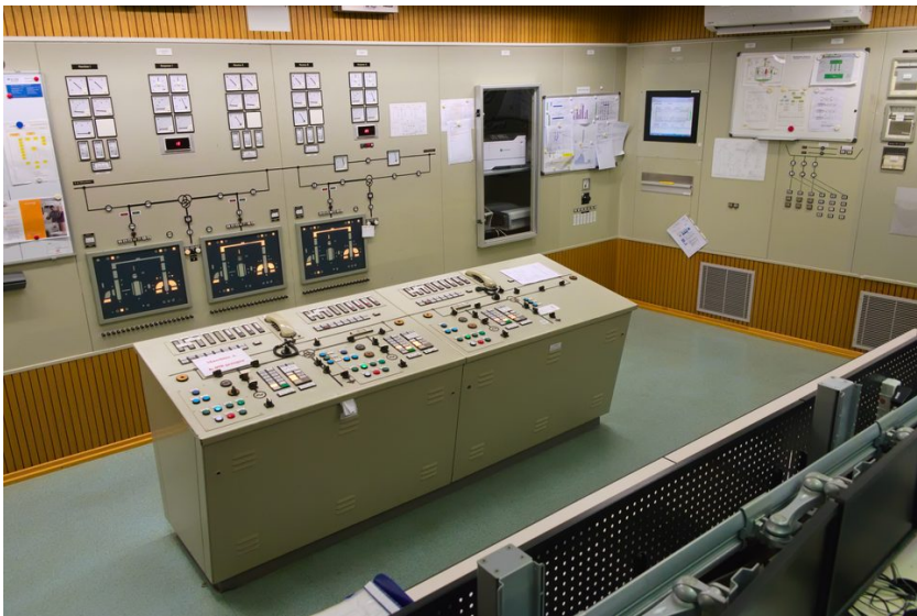
A pumped-storage power station control room.
